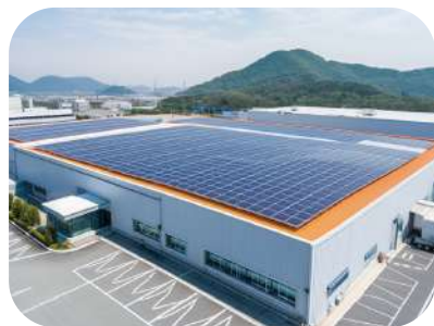
Solar Power Plant System
