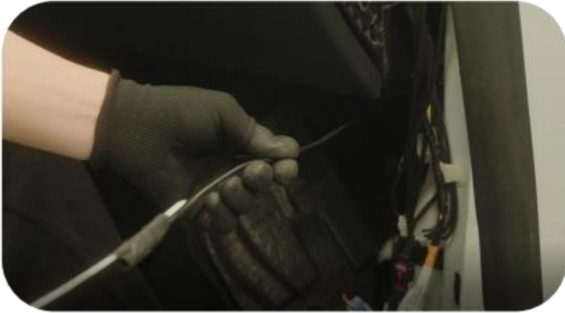
9. Pull out the wiring strap from the passenger side (Tie the wiring harness in the cabin)
