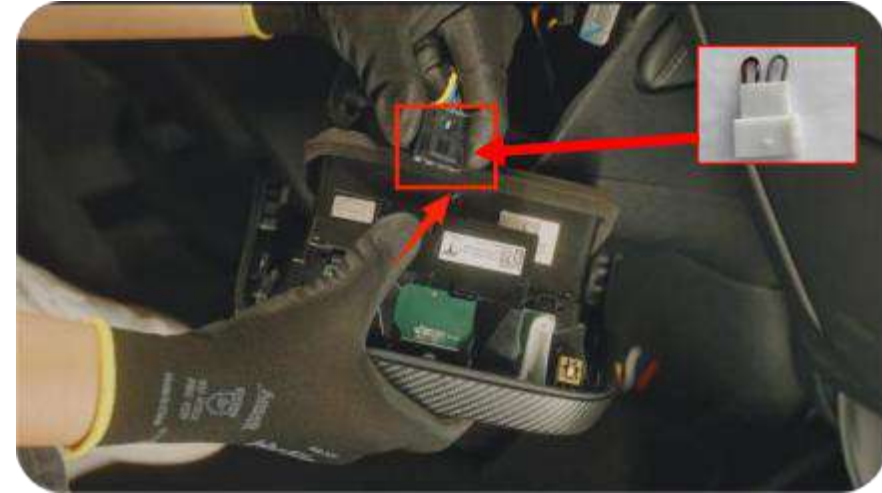
2. Pull out the plug of the charging module, and connect the emergency plug to the charging module. Electrical module plug mating
